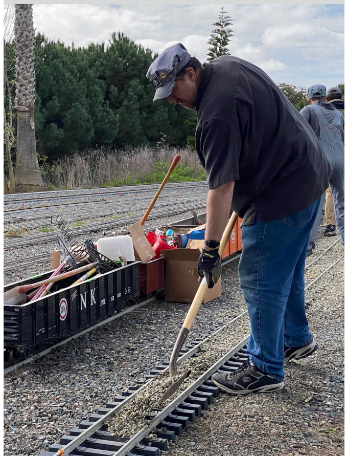
OCME VP of Facilities, Mike August works on track in Platfoot Yard during a recent work day.
